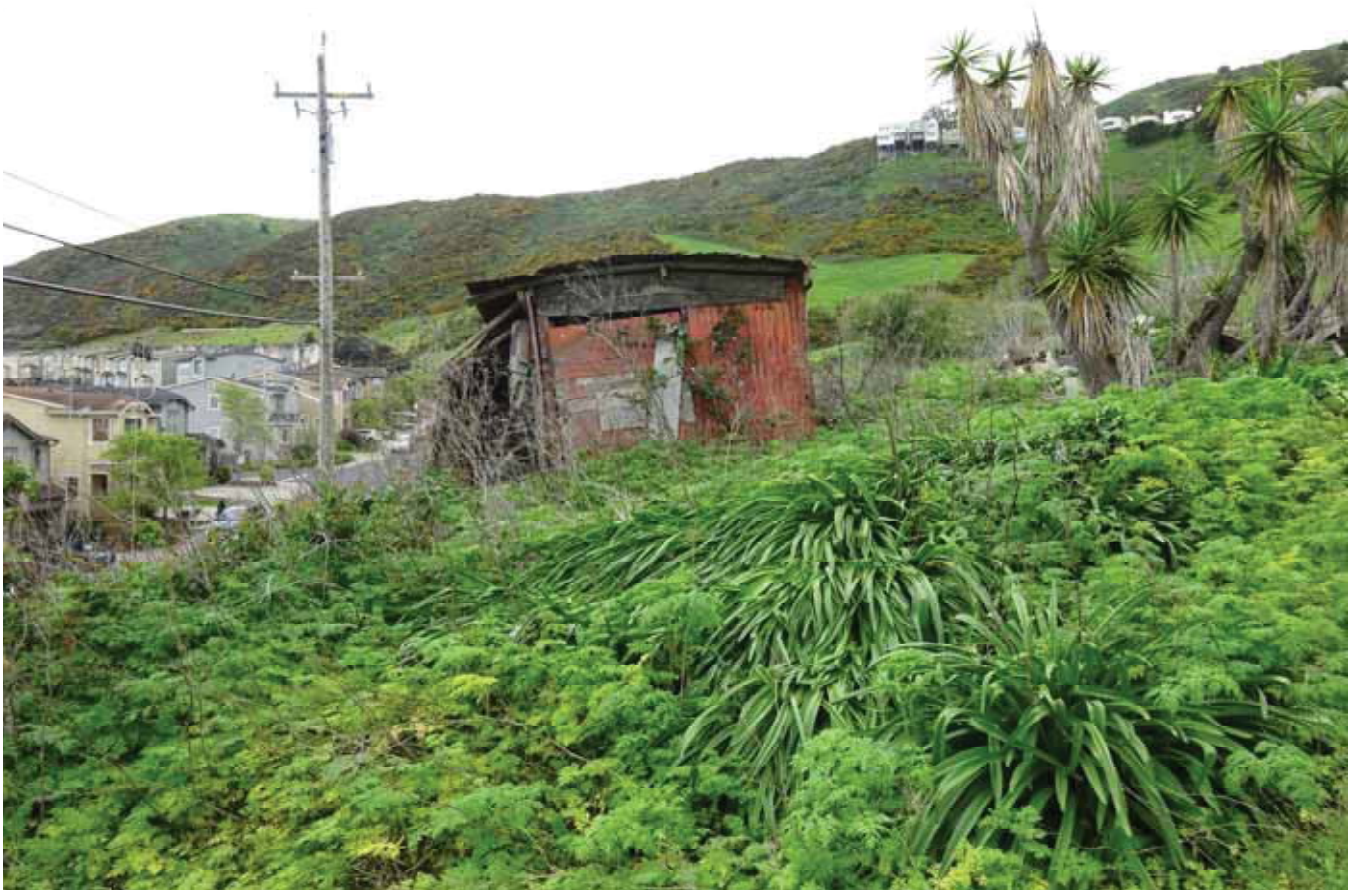
4. View of dilapidated shed on east property.
