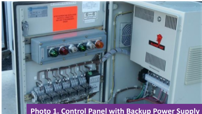
Photo 1. Control Panel with Backup Power Supply
