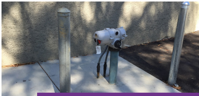
Photo 2. Motor-Operated Actuator Installed at Glenview Tank 3
