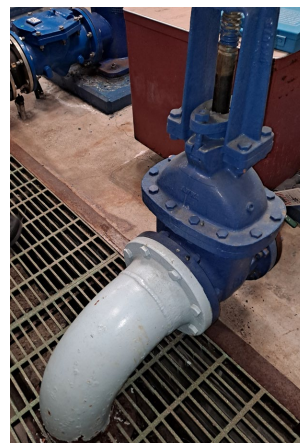
2-3b. Space for connecting third pump
